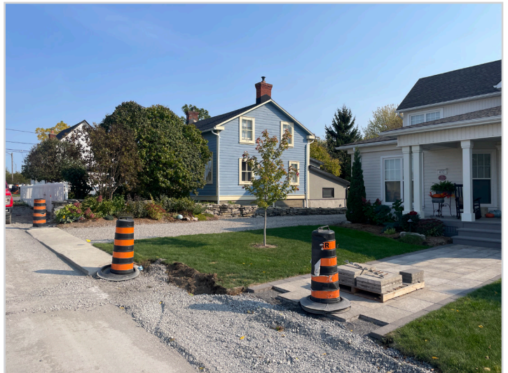
Figure 6: Looking east along Wellington Street from the frontage of the subject property.
