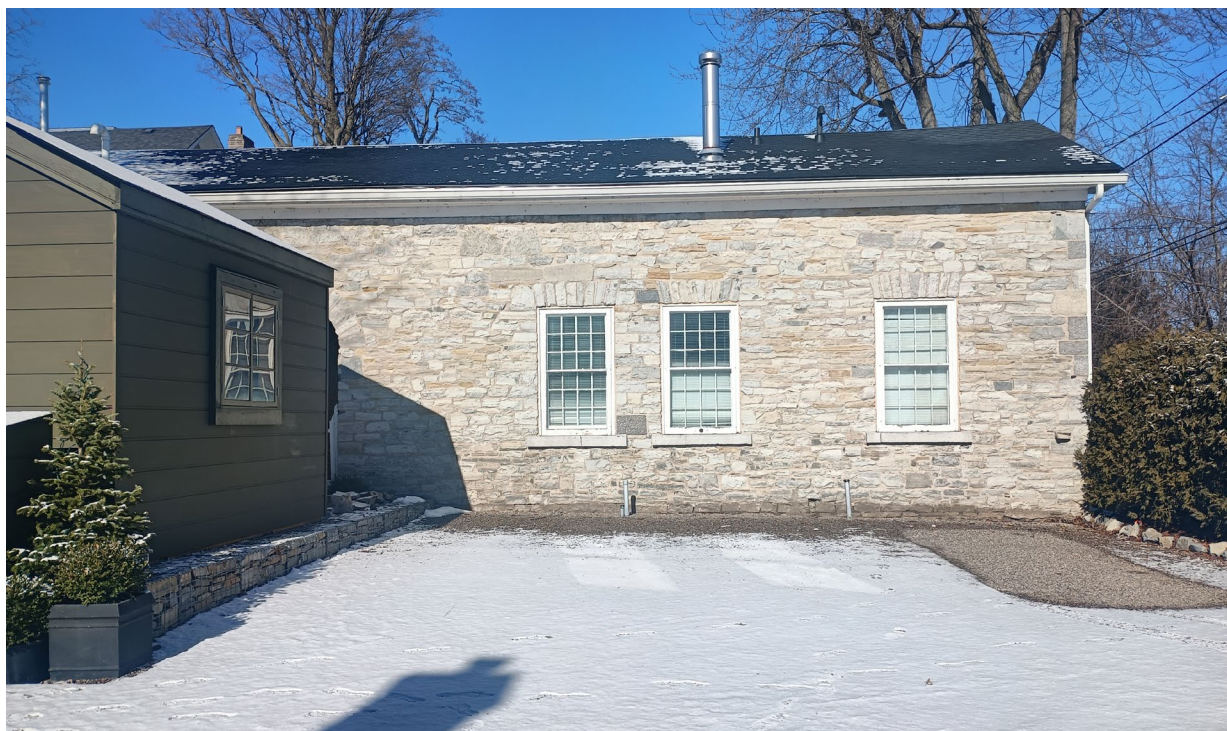
Looking north towards the east elevation of the shed and the south elevation of the adjacent stone outbuilding.
