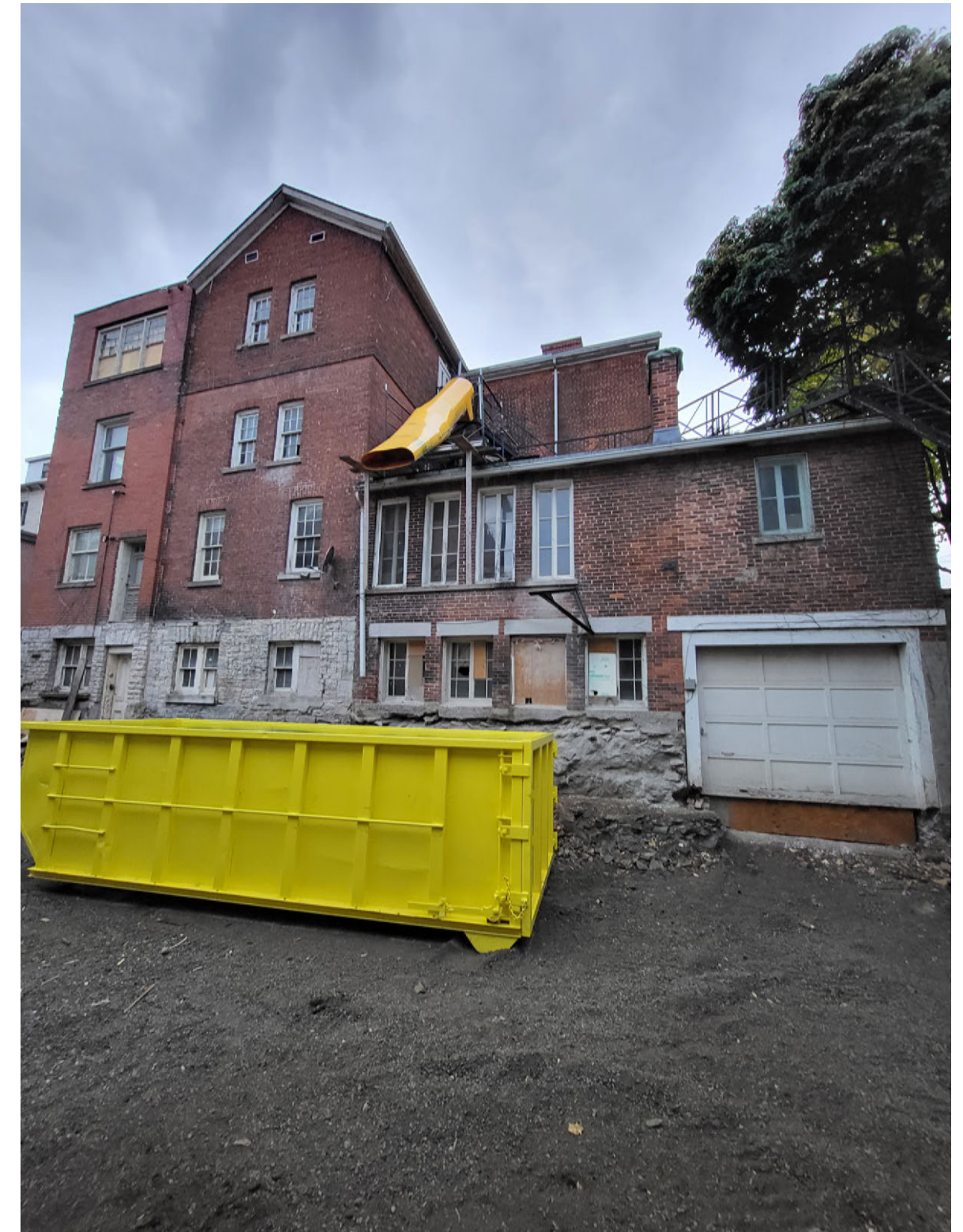
The Belvedere - Courtyard and Carriage House - Chimney to be removed 01 of 04 Shoalts and Zaback Architects Ltd. sza
