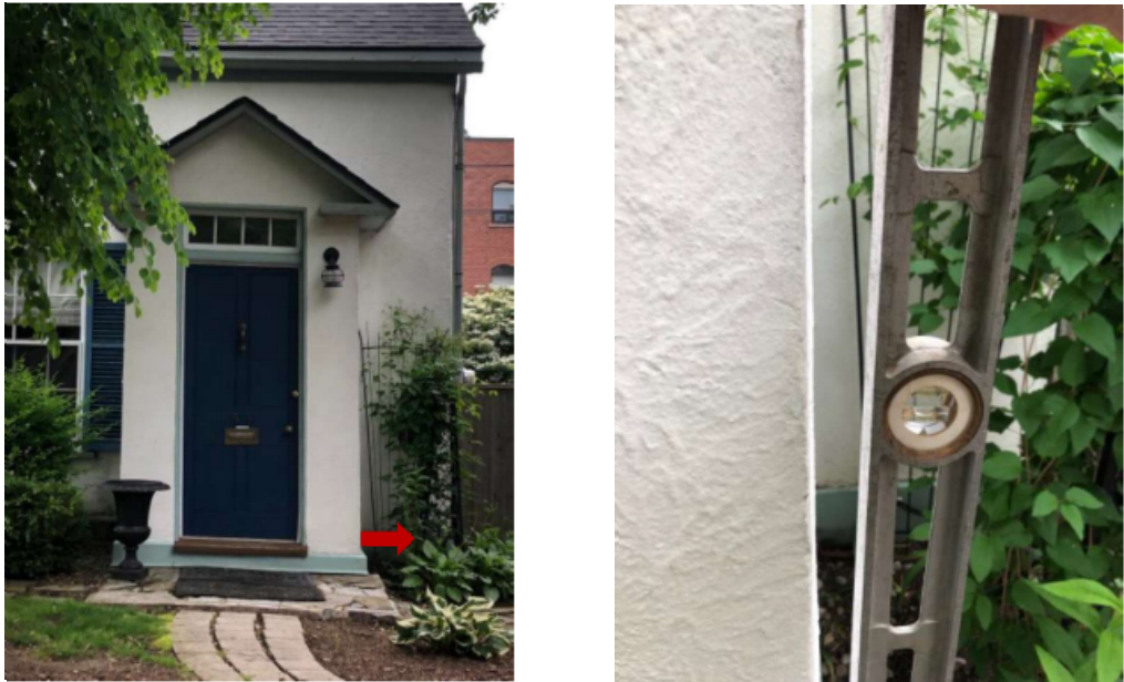
These photographs show the bottom of the side wall three inches out of plumb.
