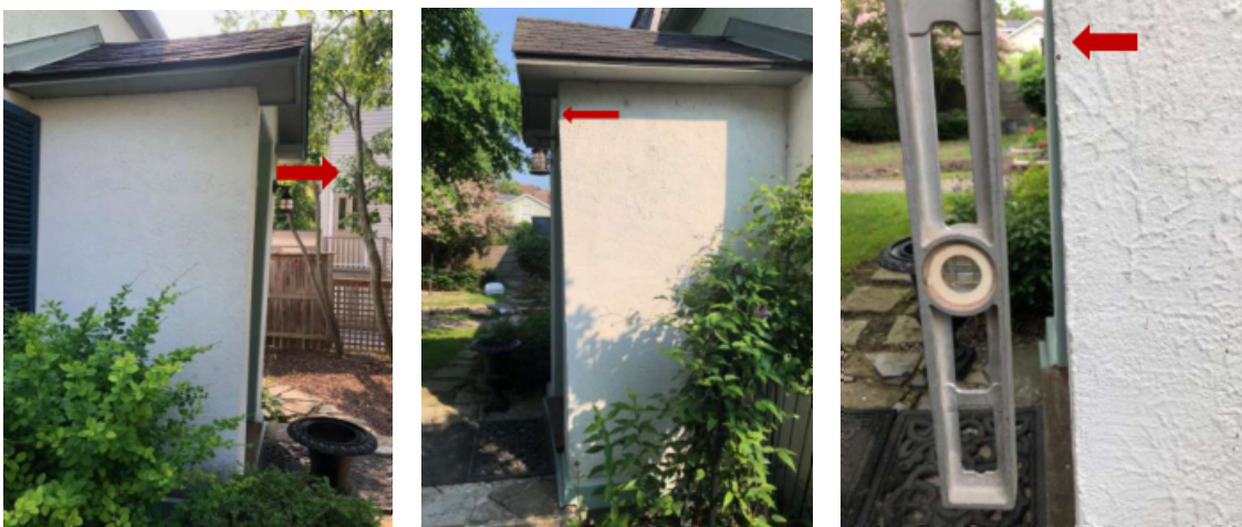
The images above show the street-facing wall four inches out of plumb. Its top leans toward the street. This is likely due to lack of a proper foundation.
