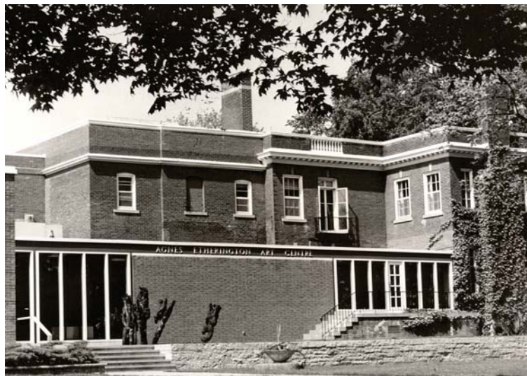
86. Archival photo of AEAC showing 1-over-1 storm windows at second floor of the Historic House
