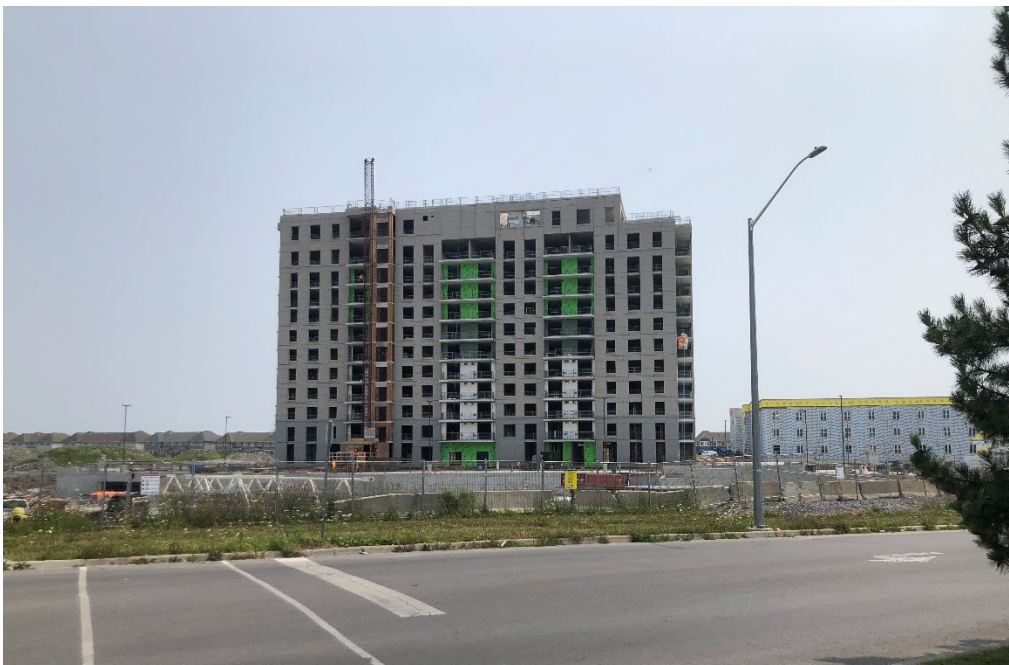
Figure 4: Looking south-east from Rockwell Drive to the apartment at 1560 Rockwell Drive and the long-term care facility at 1306 Demers Avenue (under construction).
